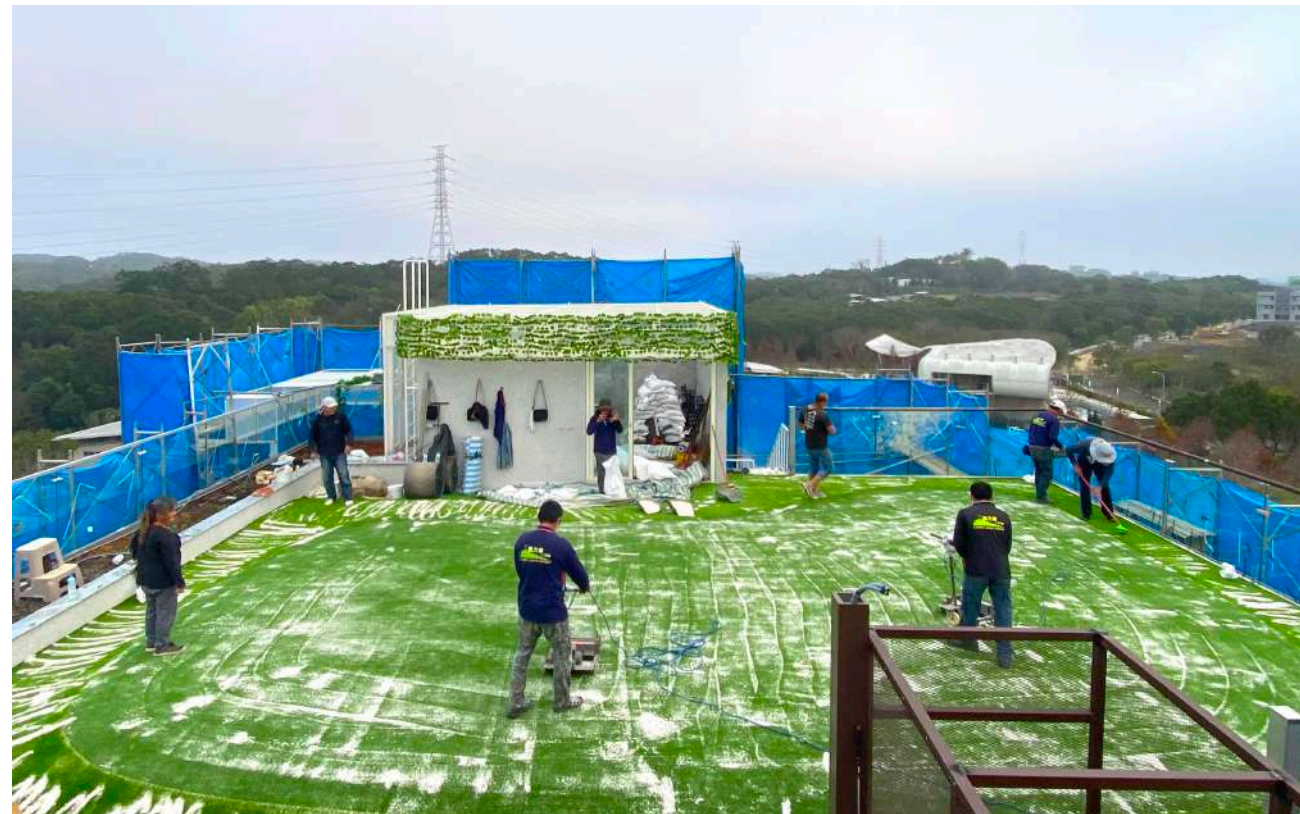
Fig. 1: Instead of any adhesive, fine sand was used to secure the turf patches in place. Fine sand is pushed to the interface between the artificial turf and the base structure to lock the two layers together.
